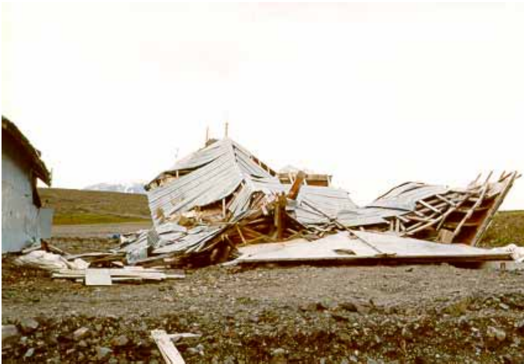
Photo 6. Snow Damage to the Camp
